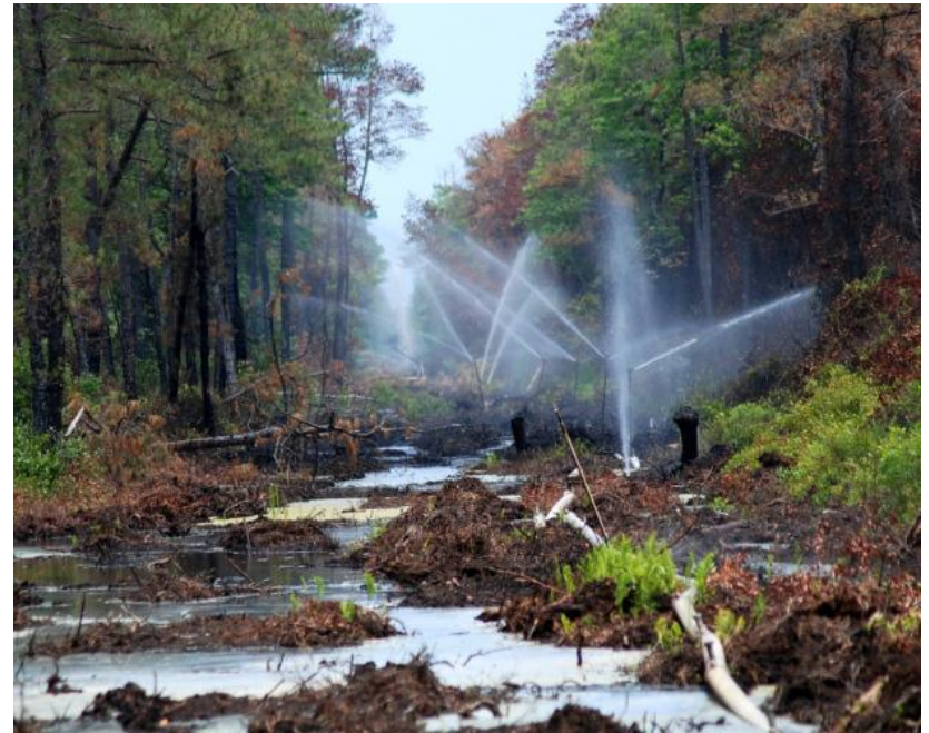
Fire Break and Sprinkler line
